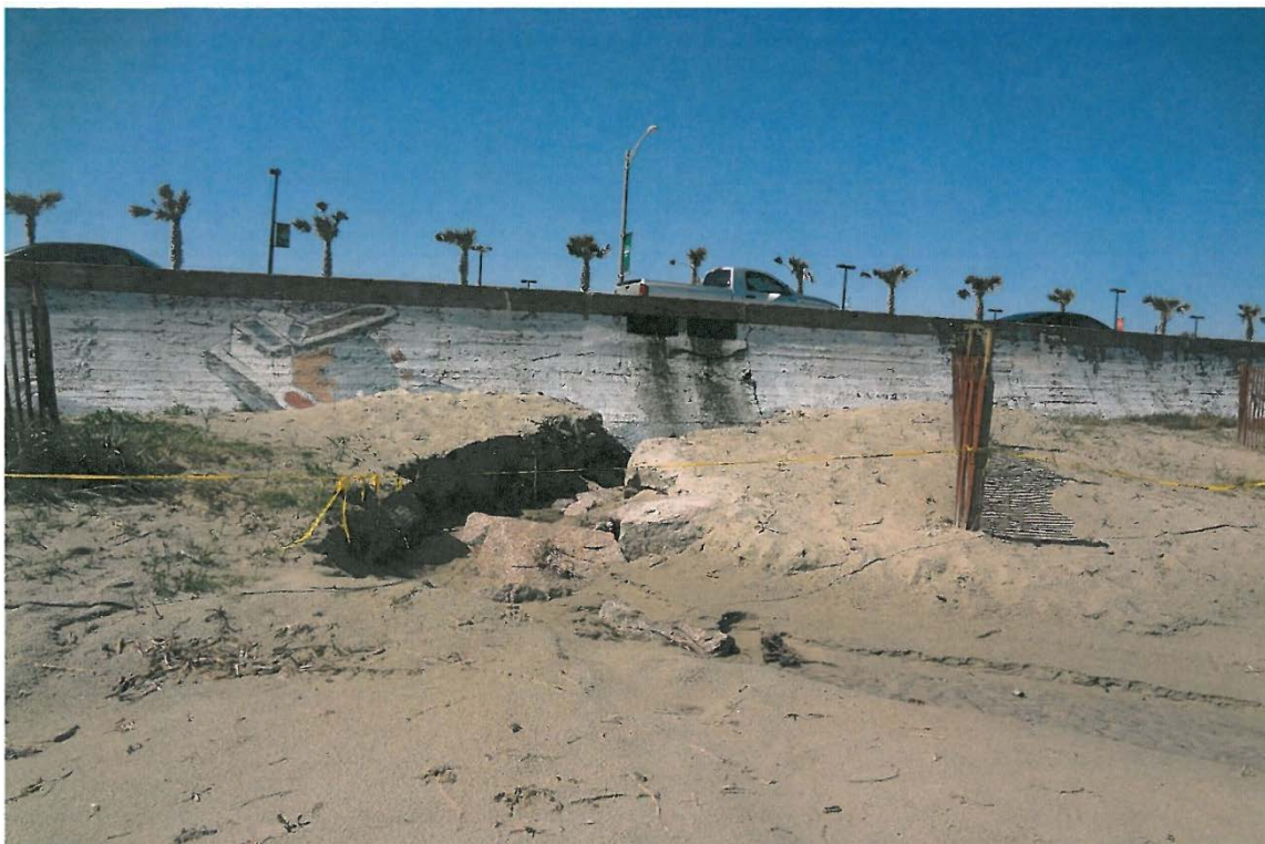
Figure 2. Photo of a runoff scour channel at a seawall drainage point on a central Galveston beach (Photo by Galveston Park Board of Trustees, accessed on: 04-17-2013).
