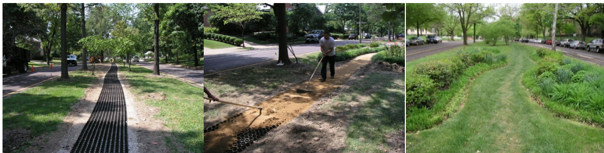
Figure 16. Photos of construction phases of a reinforced turf application for a jogging path (Source: Invisible Structures, Inc.).
