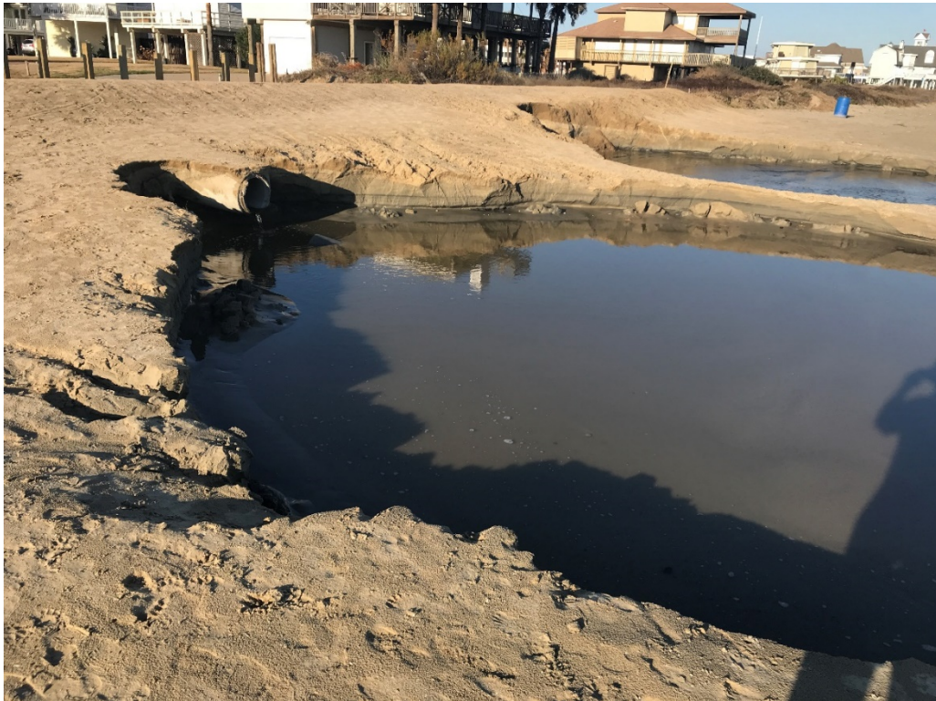
Figure 3. Photo of an example of scour holes and pipe failures at a drainage outfall near Pirates Beach (on the beach side of the dune at “Buccaneer Boulevard”; photo courtesy of Chris Robb, photo received on 01-29-2018).
