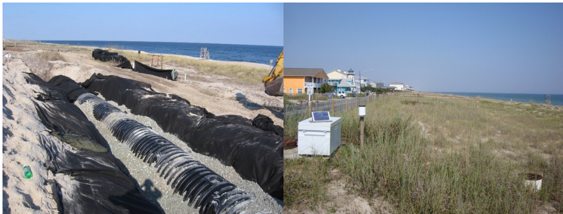
Figure 25. Photos of a dune infiltration system being installed at Kure Beach, NC (Source: Town of Kure Beach, NC).
